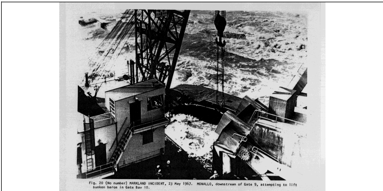
Figure C-1 - Removal of barge wrapped around dam pier - Markland Lock and Dam, Ohio River, 1967
